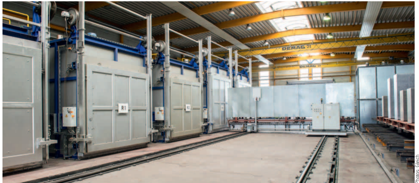
Fully automatic plant for heat treatment at Gleich
